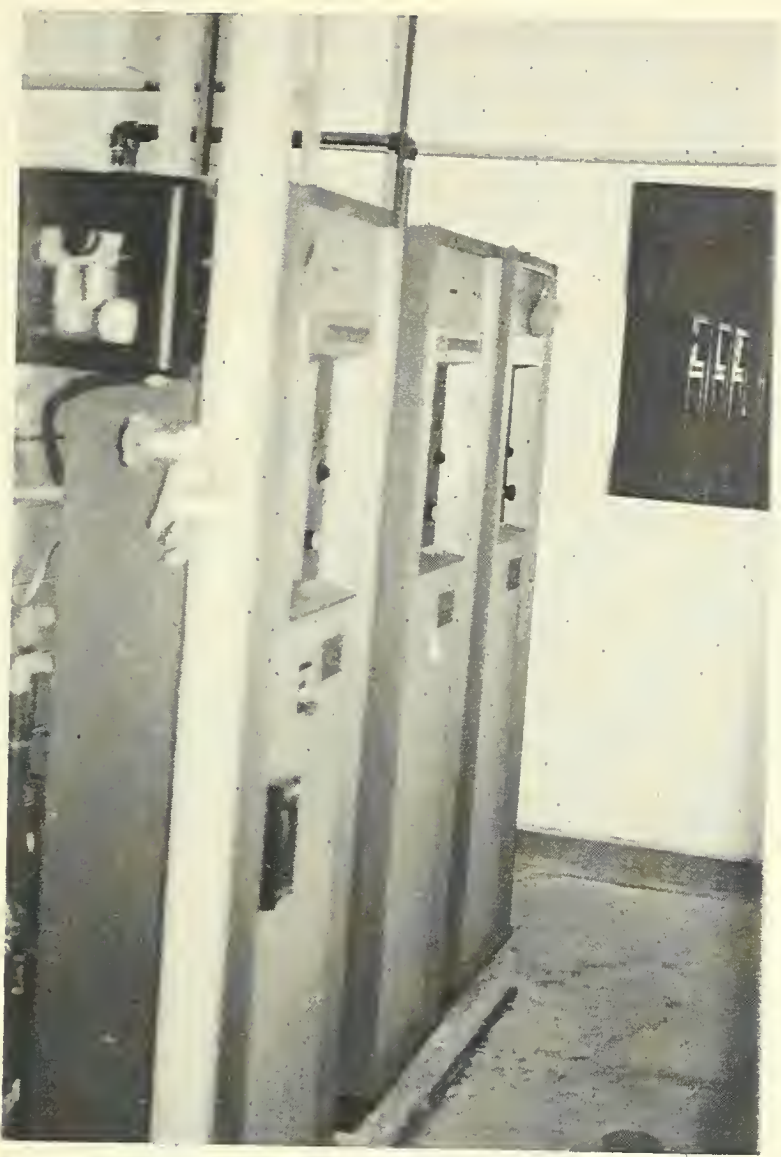
25. PRE, POST AND STANDBY CHLORINATORS
